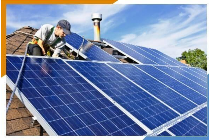
Fig. 1. The installation of solar panels (worker uses a safety harness for secure work at height)
